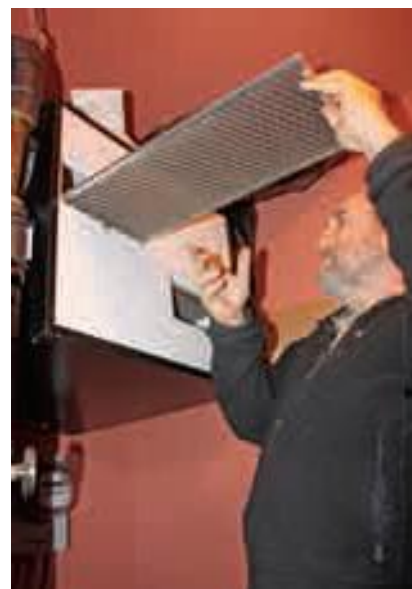
An energy recovery ventilator introduces fresh, conditioned air into the well-sealed home, with little heat loss.
