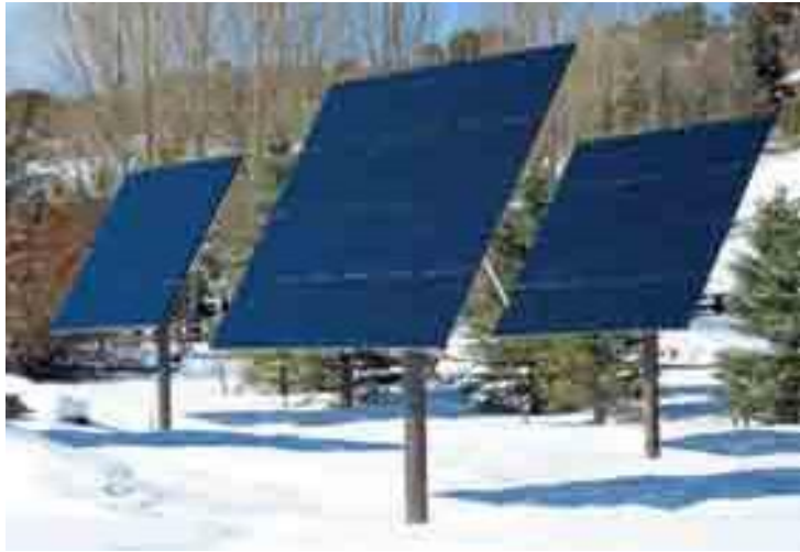
Pole-mounted arrays and trackers get the modules up off the ground, away from shading obstructions like bushes and snow.
